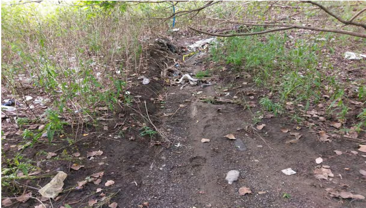
PHOTO 19: View of INT 4, looking west towards Route 7 northbound. Note refuse and sedimentation in the channel.
