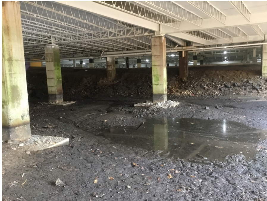
Photo 3. Portion of Wetland 3 under office building. Stantec. March 25, 2021.
